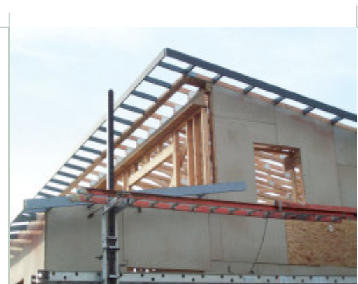
Whitmore used high-perm-rating Homosote wall sheathing to provide a breathable wall exterior; a 3/4" rainscreen will be provided
