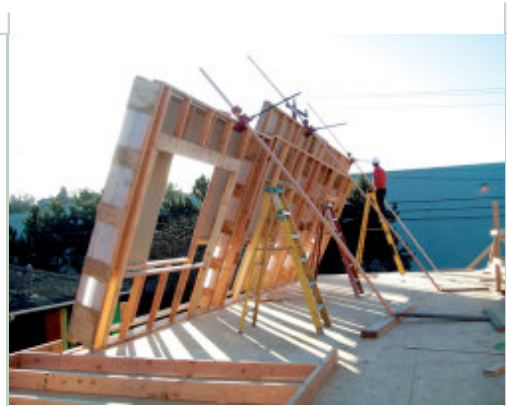
Dan Whitmore of Blackbird Builders is using a "Larsen truss" detail in this Passive House he is building in Seattle for his family. The 14" wall cavity will be insulated with dense-pack fiberglass to achieve approximately R-55.
